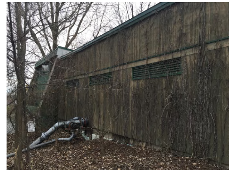
Station d'épuration, Jonathan Cha, 2016.
