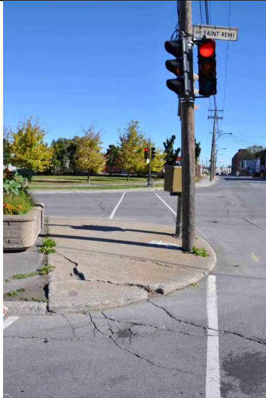
Issue 1: No curb cut-out, the median is not designed for individuals with reduced mobility
