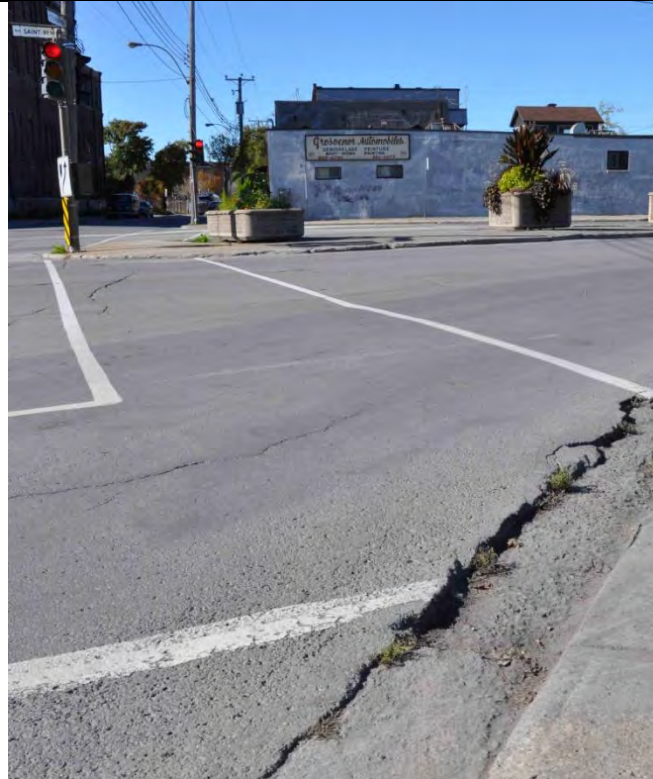
Issue 2: The curb is in poor condition, it poses a problem for individuals with reduced mobility
