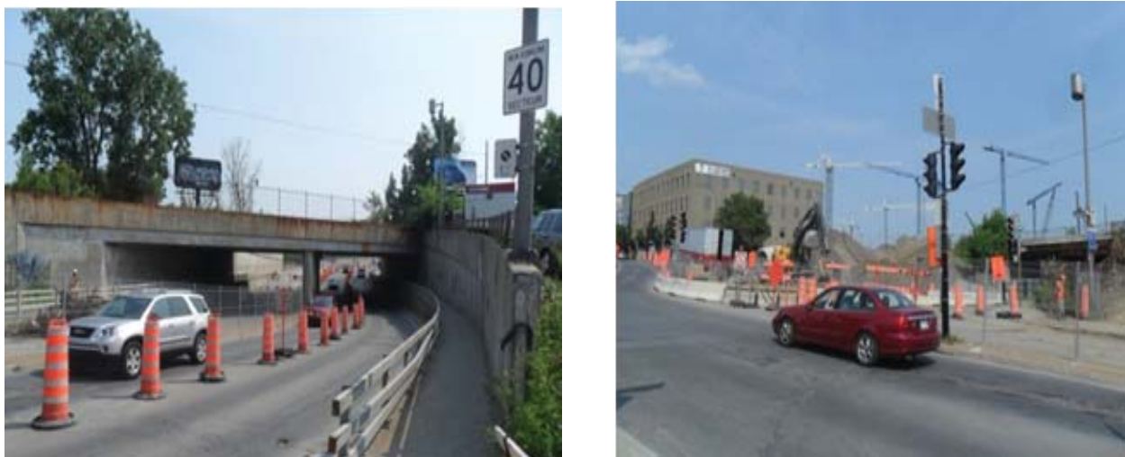
Figure 23. Décarie Blvd. and Upper-Lachine road closures and lane reductions, July 2011 Credits: Jill Merriman.
